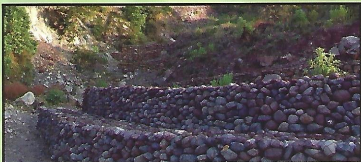
Crates & DRSM Work at Seri Mooni Irrigation Canal in Co.36/Blr of Mahanpur Range of Basohli Forest Division
